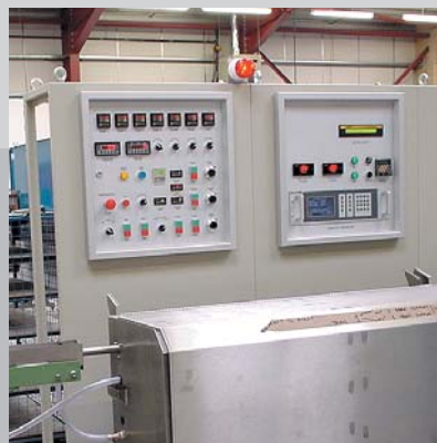
LAN Sheathing Line Control Panel
